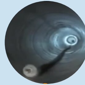
Round Duct Cleaning
